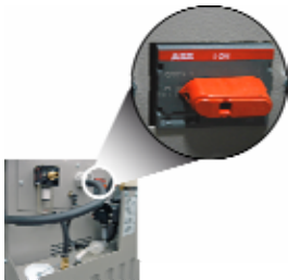
Fig. 12: Power switch (in "OFF" position)
