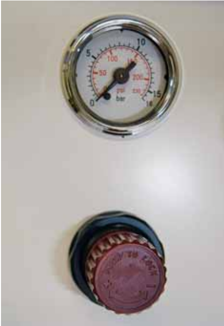
Fig.25: Pressure gauge and pressure regulator
